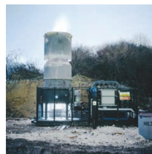
■ Figure 10.62 Deep in the waste of landfill sites, methane gas accumulates and must be burnt off or it becomes dangerous – a landfill flare-off
