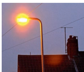
Figure 2.34 A sodium street lamp
