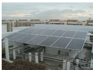
■ Figure 9.27 Solar cells on top of government-built flats in Singapore
